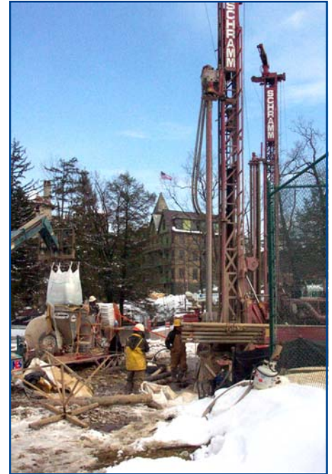
An important preliminary step in installing geothermal systems is drilling deep wells in an area close to the building.
