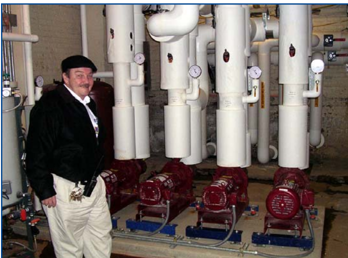
John Clausson stands in what used to be Bowne Hall boiler room, which has been outfitted with geexchange pipes.
