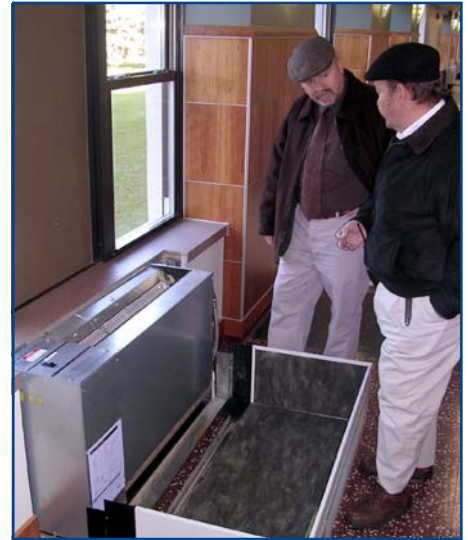
John Clausson, right shows Marketing Representative Kevin Smith how registers are used for both heating and cooling.
