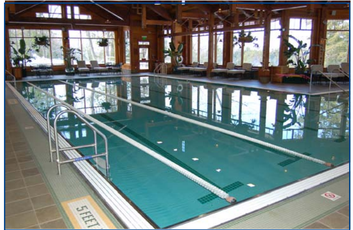
Geexchange technology keeps the pool area heated and regulates humidity.
