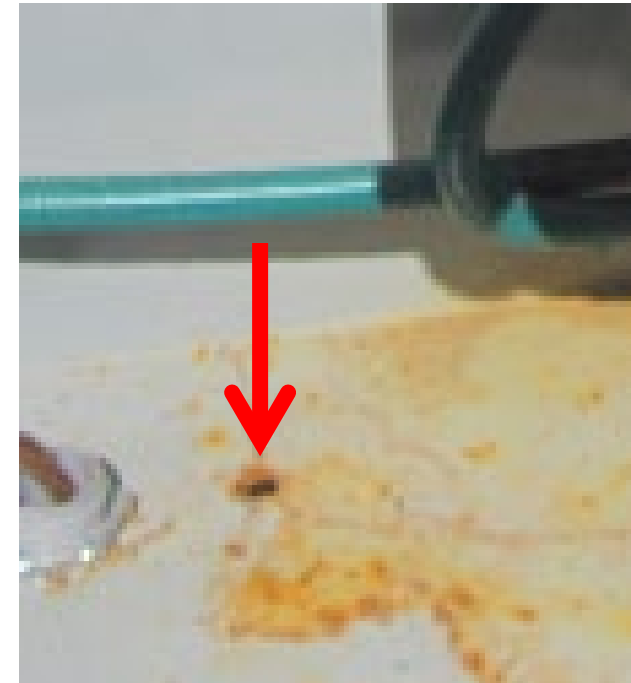
Weep hole doing its job. Notice where water line ends.
