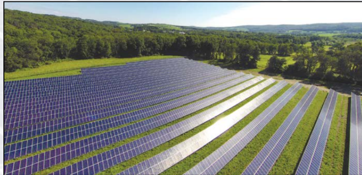
Remote Net-Metered 1.368 MW Solar PV
